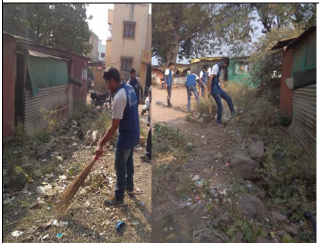
Cleanliness and repair of streets
